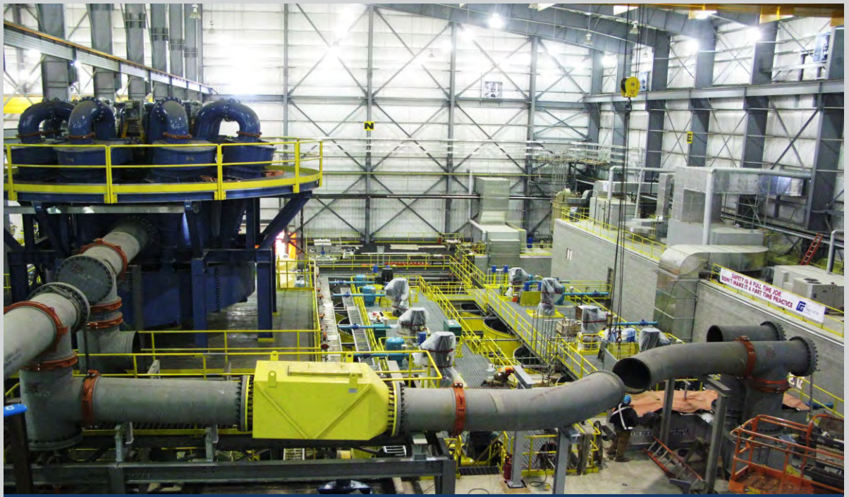
Cyclone and Flotation Circuit
