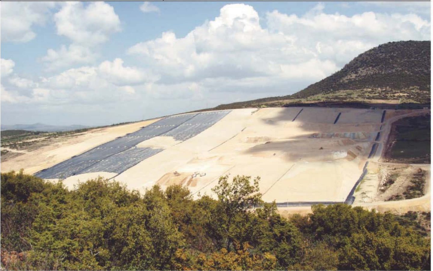
Vancouver, British Columbia-based Merit Consultants provided construction management services for Eldorado Gold Corp.'s Kisladag Gold Project in southwest Turkey.
