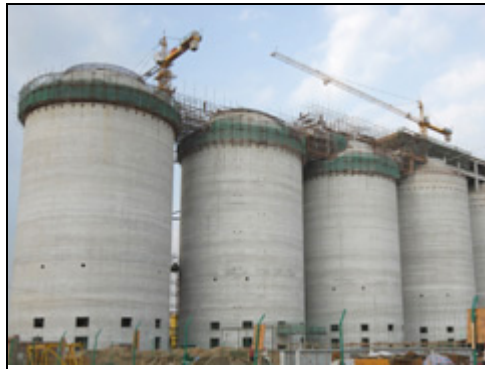
Raw Coal Silos
