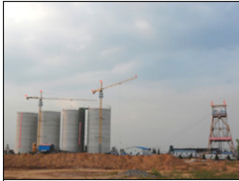
Raw Coal Silos
